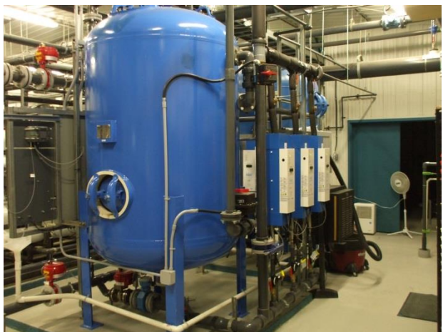
The New Sand Filter with UV
