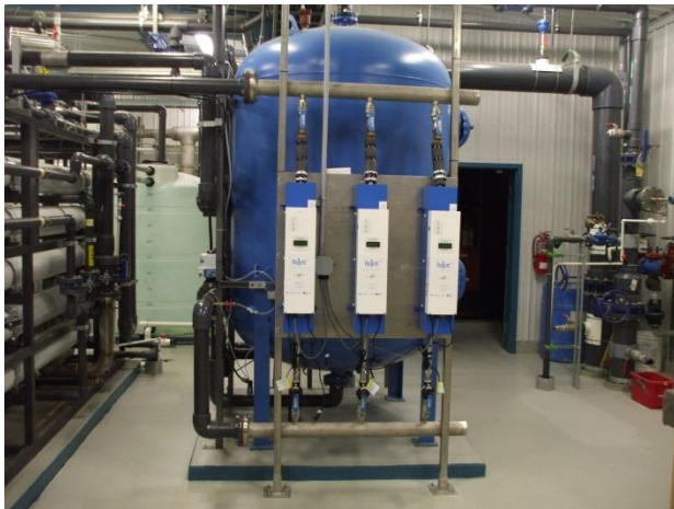
The Original Sand Filter with UV upgrade
