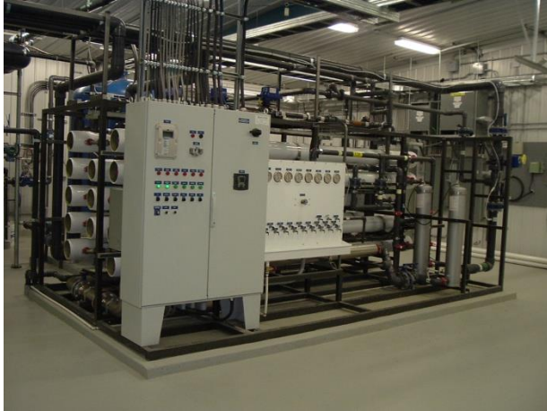
The South RO (original unit)
